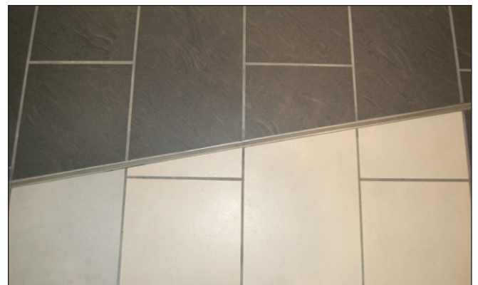
For this lobby, a membrane allowed installers to place tile movement joints in locations other than directly above control joints in the slab. The joint profile was placed along one of the curves to create a natural-looking break between the two different colors.
